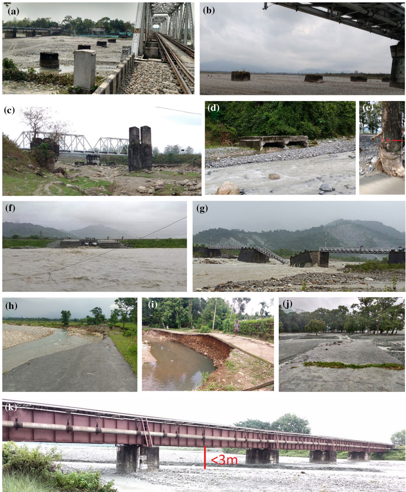
Fig. 8 Some signatures of destruction by the flash flood: Along with almost all the rivers of Jalpaiguri District. a Chel, b Diana–Chamurchi, c Ghatia, d Lish river bridges were destroyed in the flash flood of 1968, e more than 1 m sediment was removed by the flash flood in Ramthi river in 2011, f flash flood in Ramthi river, 2019, g bailey bridge in Samtse, Bhutan collapsed in July 2016 due to flash
